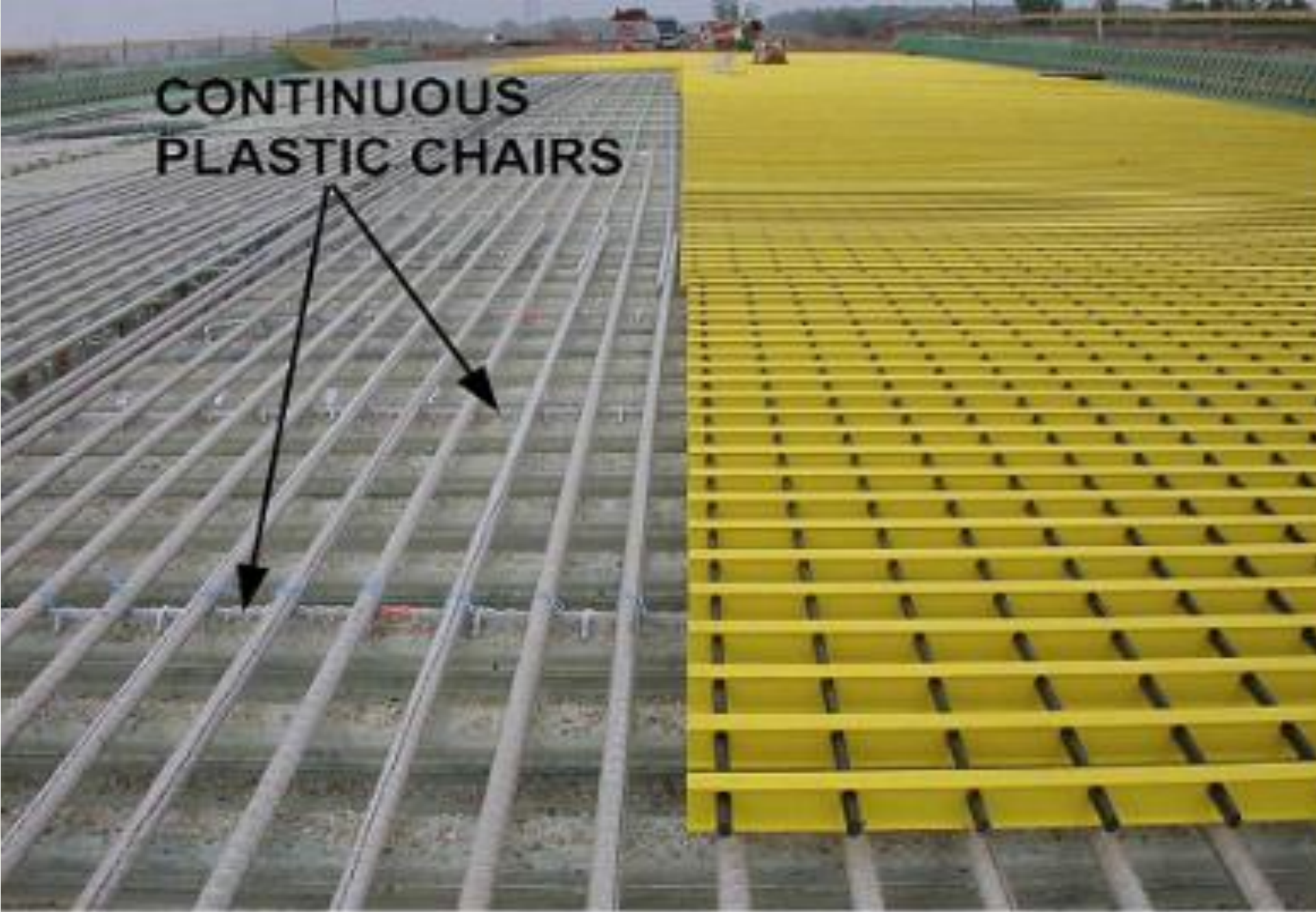
Fig. 12. SIP FRP deck panels, FRP rebar, and bi-directional FRP grid during placement.
